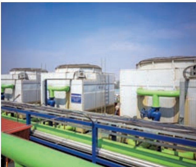
Cooling towers at Biocon Park, Bangalore
