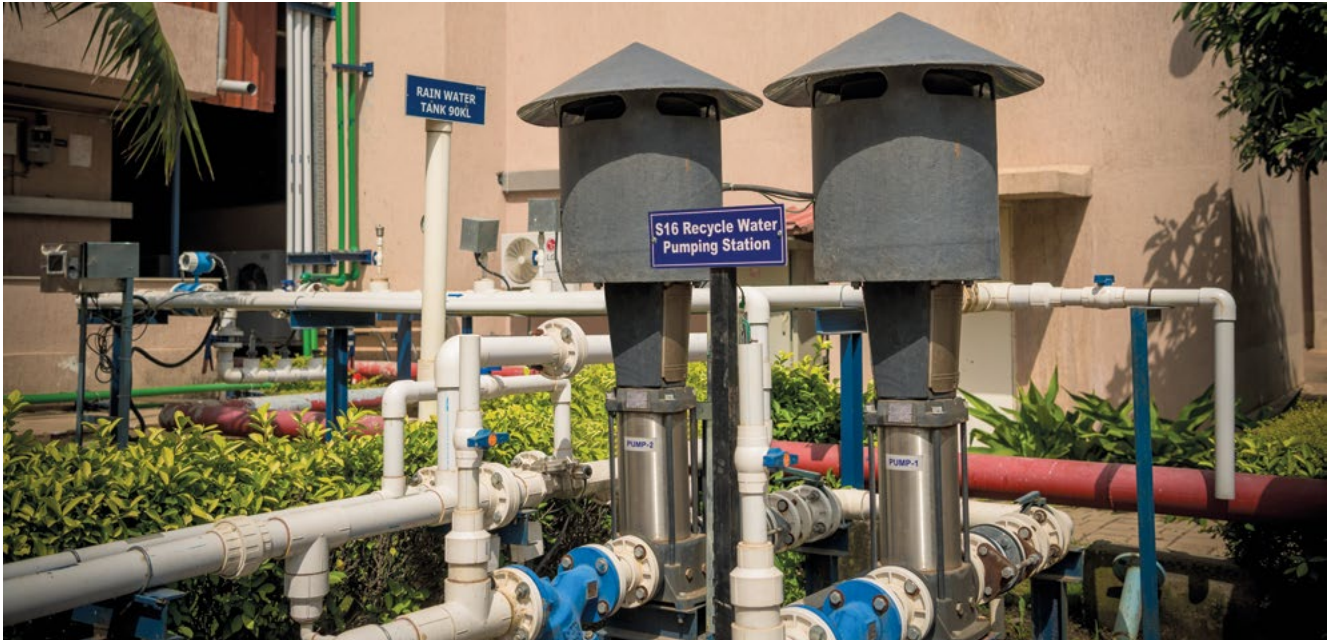
Recycle water pumping station at Biocon Park, Bangalore
