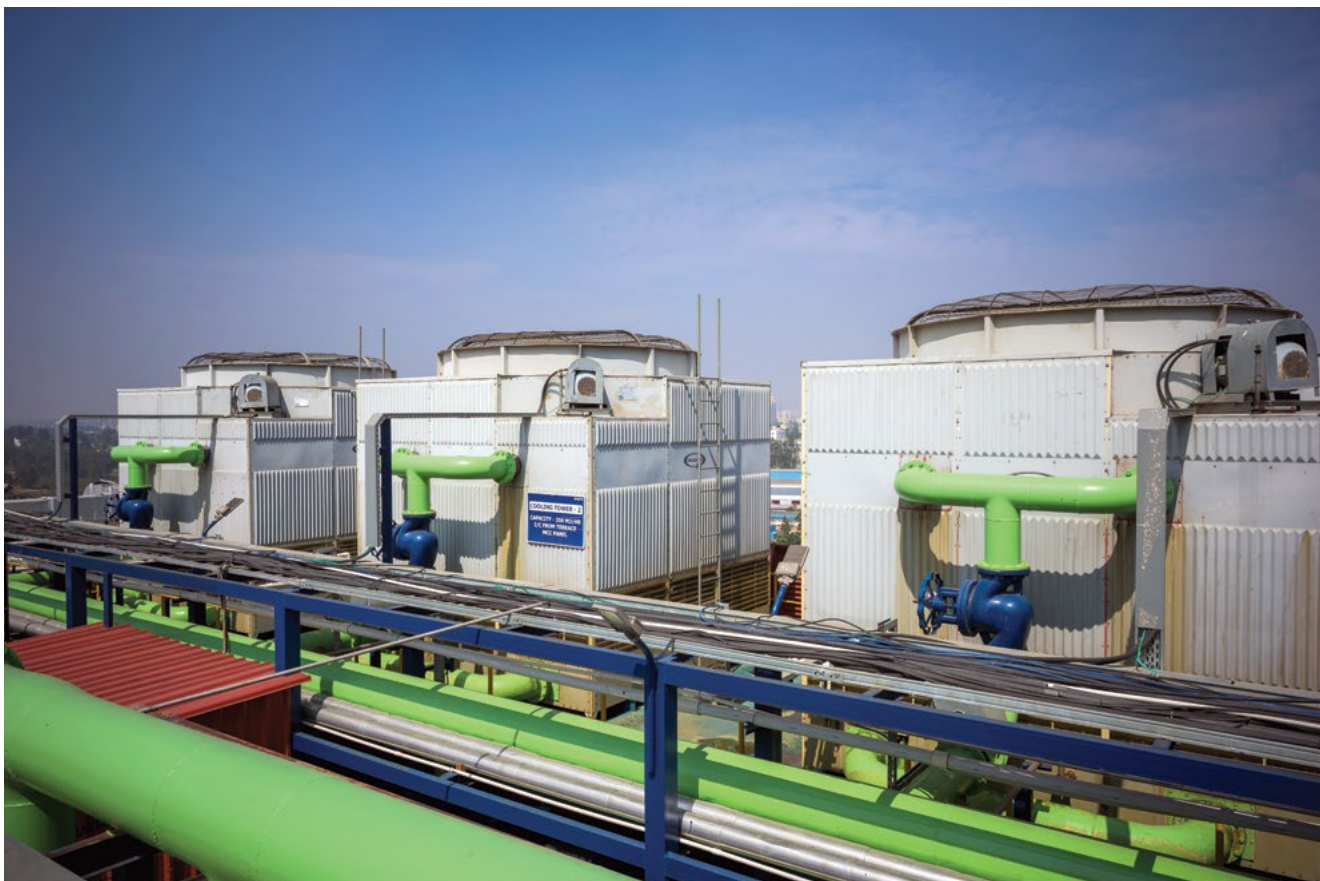
Cooling towers at Biocon Park, Bangalore
