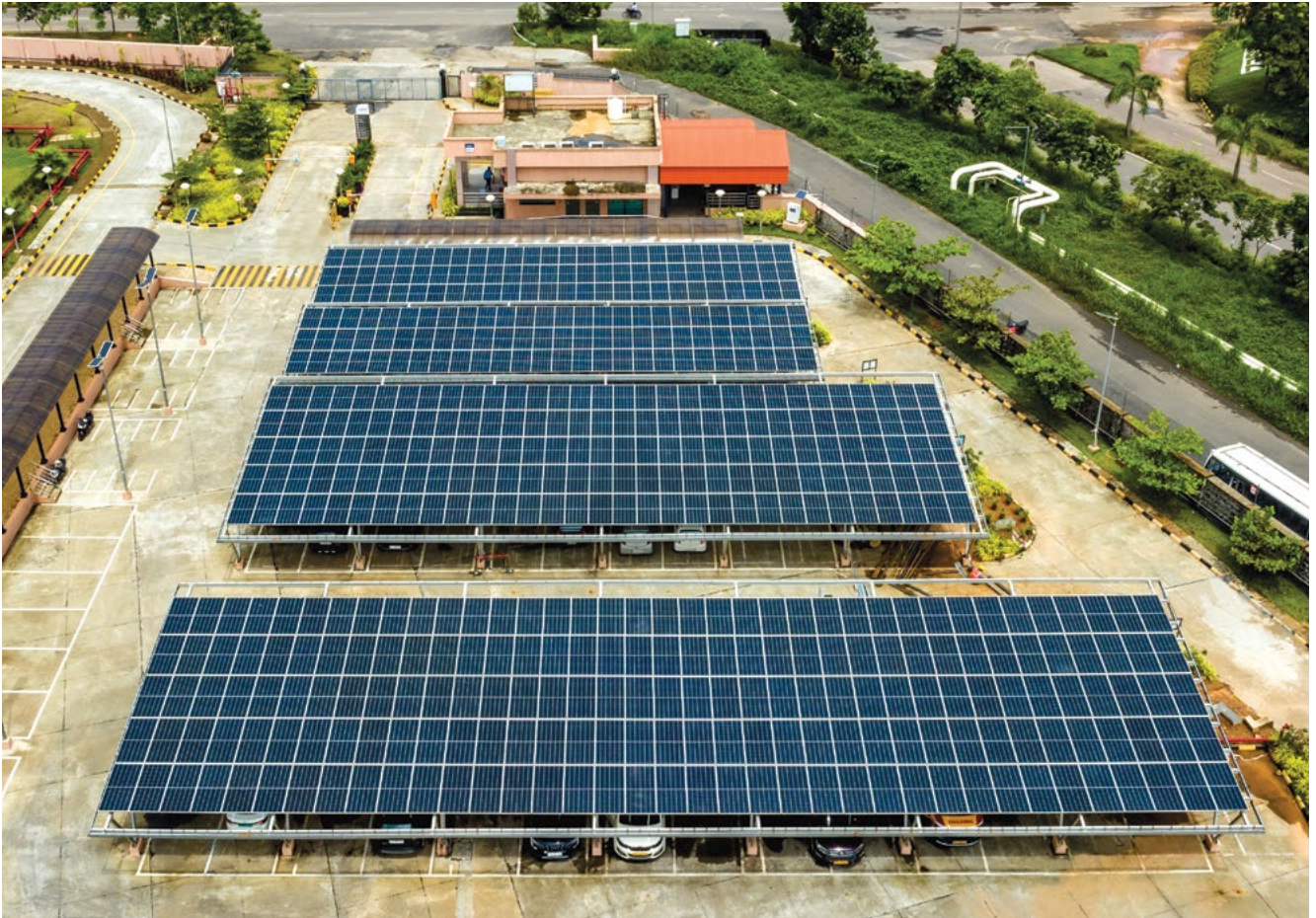
Carport solar panels - Mangalore campus
